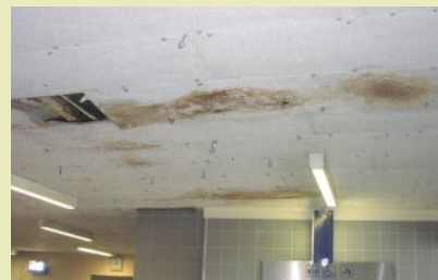
Lekkagesporen in de stationshal
